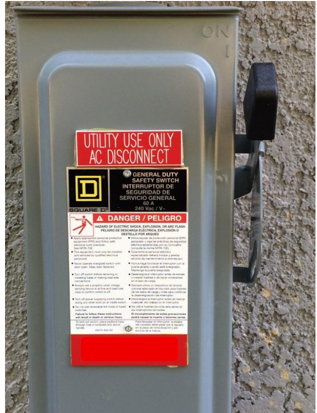
Figure 3: Utility Use Only AC Disconnect Placard
