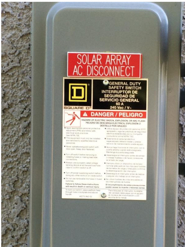
Figure 2: Solar Array AC Disconnect Placard
