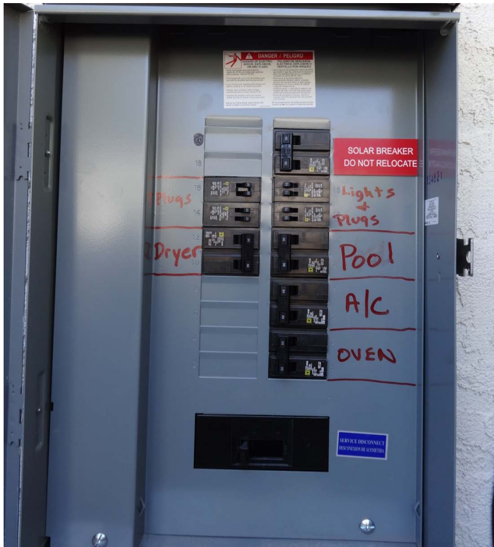
Figure 5: Solar Breaker Placard
