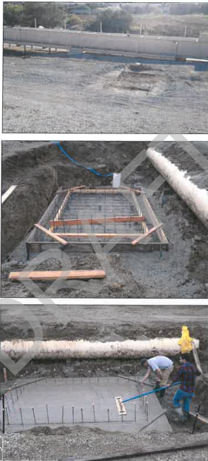
Figure A-3. Initial construction of main spill box that the meter gate pipeline drains into.
