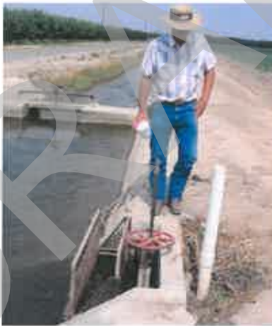
Figure B-10. This stilling well is properly located, but it has too small a diameter. The operator also needs to know the elevation difference between the top of the stilling well and the gate frame, which requires an extra computation to determine the difference in head across the gate.
