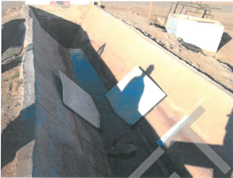
Figure 3. Side contractions rather than a traditional "Replogle Flume". Designed by USBR, Yuma. The rocks are not part of the design.
