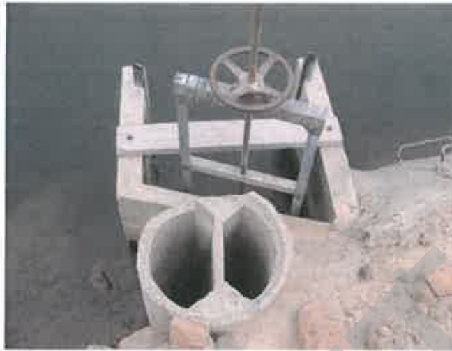
Figure B-9. An old type of dual-stilling well commonly found in Central California irrigation districts. One stilling well was connected to the canal, and the second was directly over the discharge pipe. The idea of measuring down into both stilling wells from the same center point was good, but the top of the stilling well was so close to the ground surface that road maintenance quickly filled these stilling wells with dirt. Also, the side connection between the canal stilling well and the canal itself was too difficult to clean.
