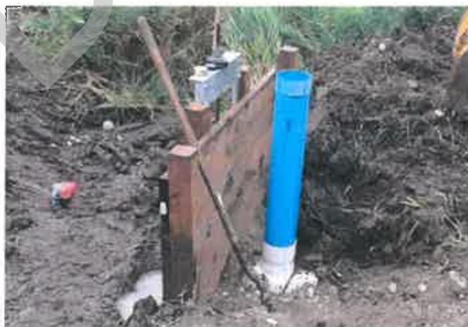
Figure B-8. Stilling well installed on an existing discharge pipe. It is constructed of PVC pipe that is too thin for long life, but it serves as an example of the correct diameter, position, and height.
