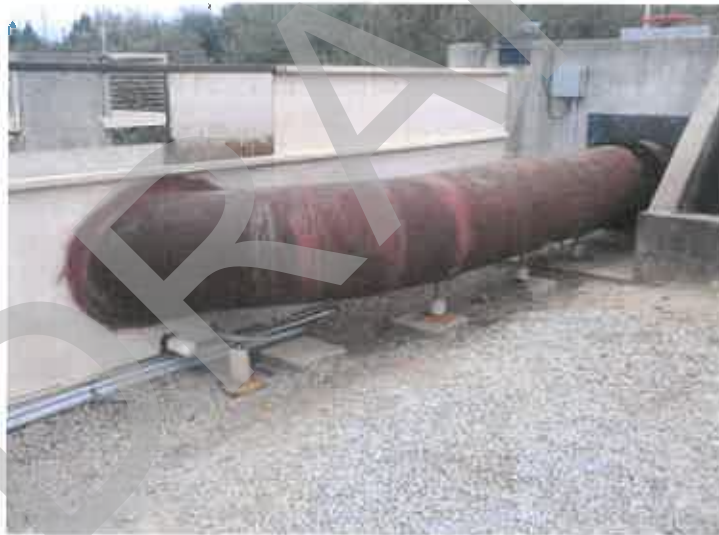
Figure A-1. Adding a 30" pipe to the head of the flume to increase the capacity into the flume (left)
